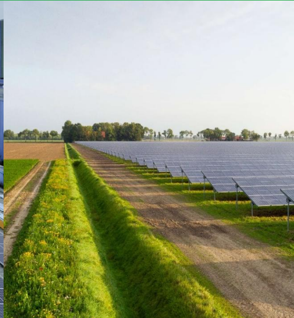
Ground Solar Power
