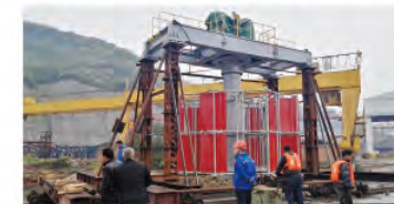
100kW门板式潮流能发电系统 100kW door-type tidal current power generation system
